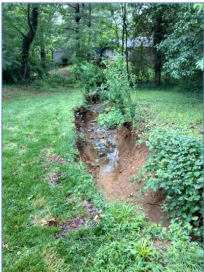
Heavily Eroded Channel (Before)
